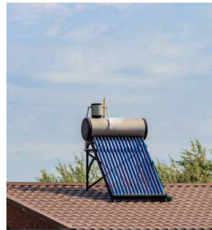
SOLAR WATER HEATERS
